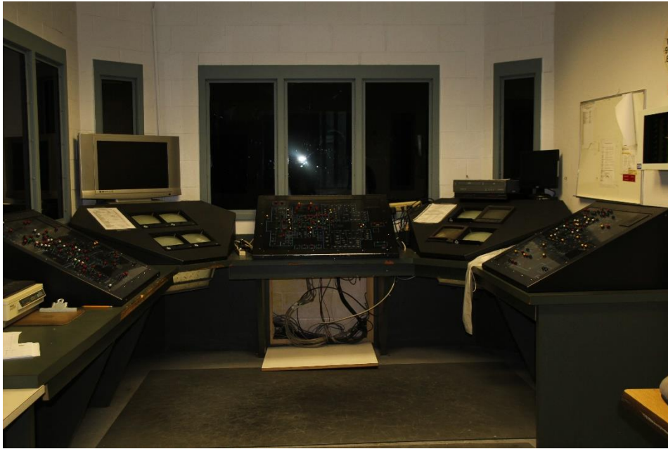
Nashville Central Control Room
